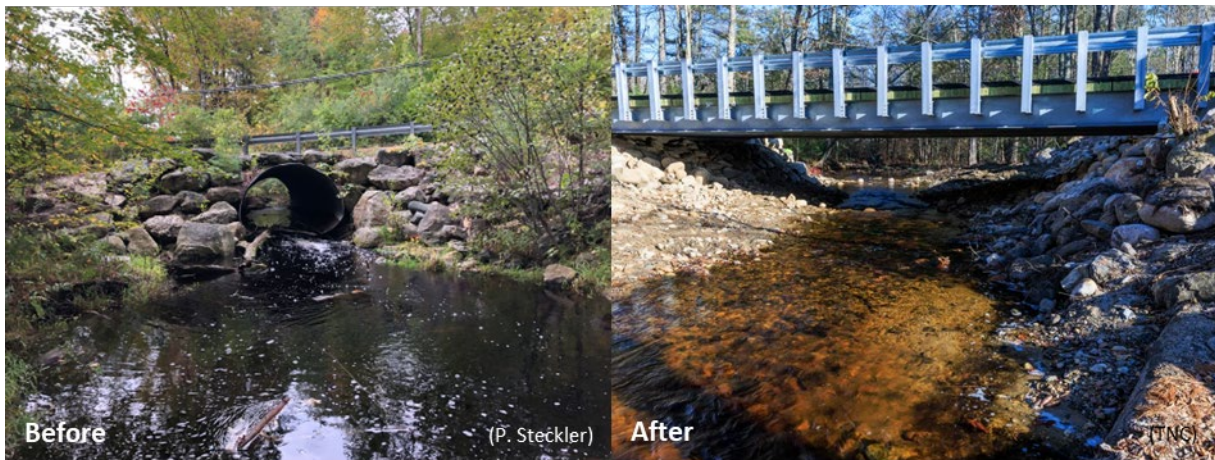
Figure 15. Before and after photos of the project site where the Oyster River passes under Topaz Drive.
