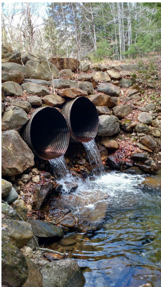
Figure 13. Perched culverts impede AOP.
