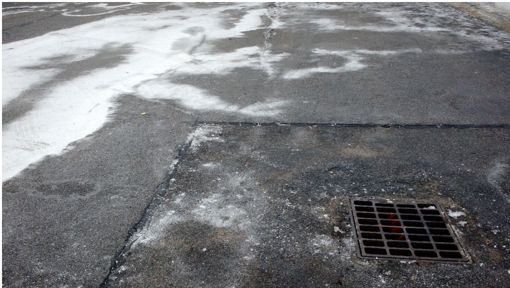
Figure 16. Excess de-icing materials enter surface waters through stormwater runoff.
