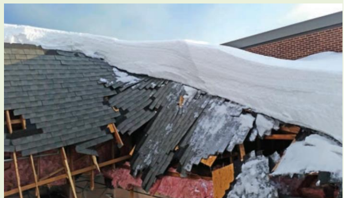
Figure 3. Partial roof collapse at an elementary school due to snow load (Building America Solution Center / U.S. Department of Education).
