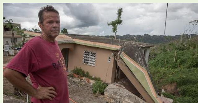
Figure 6. Home destroyed by a landslide following Hurricane Maria (Andrea Booher / FEMA).
