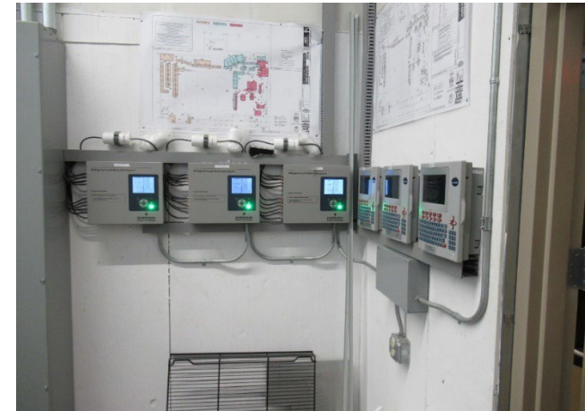
New Leak Detection System
