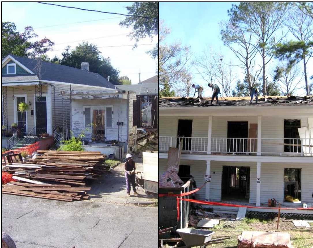
Deconstruction job training pilot projects were conducted on various types of buildings by Mercy Corps and other nonprofit organizations after Hurricane Katrina. (Photos: Brad Guy)
