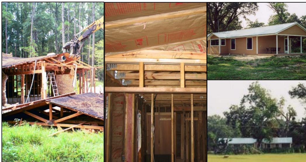
Panelized deconstruction was used to deconstruction a home in a floodplain buyout in Alachua County, Florida, and the lumber was used to build new Section 8 affordable housing inland. (Photos: Brad Guy)
