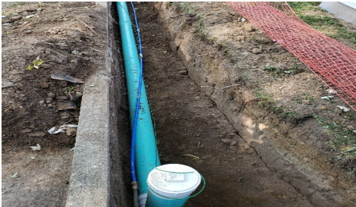
Photo #3: View of new sewer lateral and new water line (3/4-inch blue PEX tubing) at a private residence
