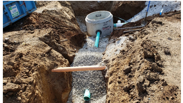
Photo #4: Looking south at new sewer structure #7 & lateral/main going north to old MH #250056
