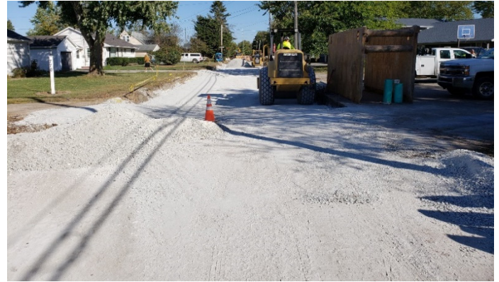
Photo #2: View looking east along Hamilton Avenue during preparation of the road bed base
