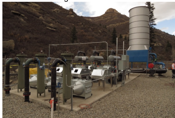
Combustor and one of three 1-MWe power generators being placed at Elk Creek mine (compliments of Vessels Coal Gas)
