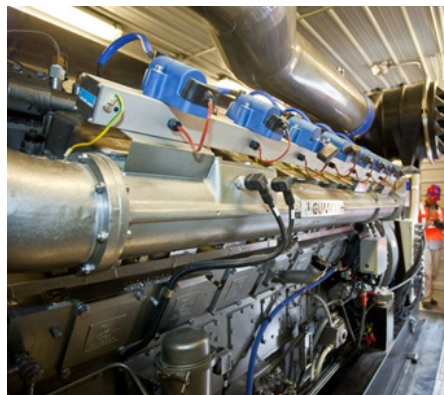
Guascor Gas Generator at Elk Creek Coal Mine Methane Destruction and Utilization Project (compliments of Aspen Skiing Co.)
