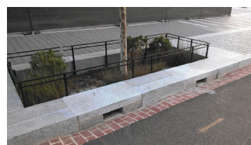
Stormwater runoff flows through roadside curb cuts into a sidewalk bioretention planter.
