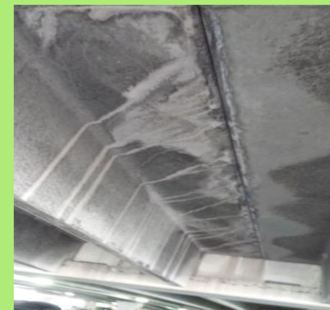
Fig. 3 Stalactite formation underneath parking deck caused by lime weeping; The PV canopy will greatly reduce water on the parking deck and eliminate need for salt.
